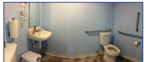
(June 2020) A panoramic view of the completed handicap accessible restroom. About $35,000 plus countless hours of volunteer labor has been invested in the renovation work. Large donations came from Valley, Perry Valley & Red Lion Granges. (Photo Credit: David Troutman)
