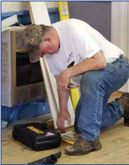
(June 2020) State Grange president Wayne Campbell, along with members from several other Granges, tackled the job of installing beautiful new laminate flooring. (Photo Credit: Beth Downey)
